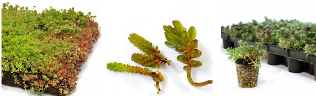
Figure 3.26 Installation methods of plants. From left to right, sedum mat, cuttings, plugs
